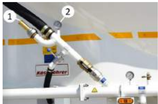
Pressure relief valve and manometer
